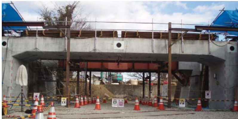
Figure 3. A full-scale model of GRS integral bridge completed in the beginning of 2009 (this picture was taken during lateral cyclic loading tests in the beginning of 2012).
